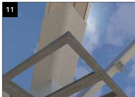
11 Measure and fit the standard valley undercladding NVU-V between the eaves and mark 'C'. Scribe to suit.
