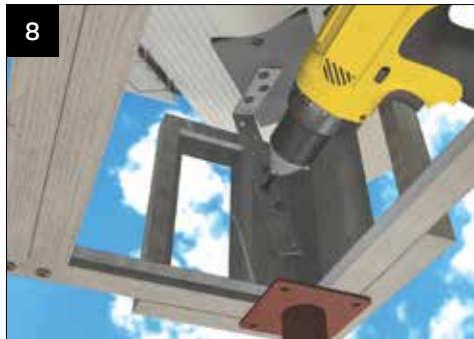
8 FIT THE STRAP CHA018 USING M4x13 SELF DRILL SCREWS, to the valley corner infill panel and the valley fixing plate. It may be necessary to bend CHA008 to suit.
