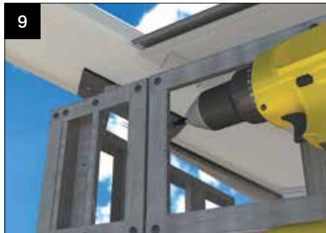
9 Fit the vertical frames. Fix the frames into the valley corner infill and the horizontal frames.
