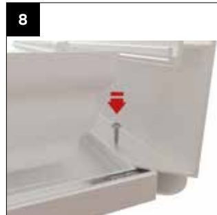
8 Offer up the middle Cornice section into position, secure using fixings provided FSD-42-19. (Long reach driver required).
