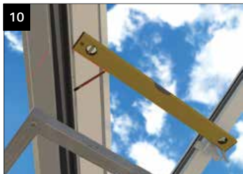
10 Using the bracket positions, level through and mark off the valley marked 'C'.
