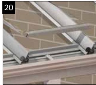
20 At this point the roof should be glazed. Any ridge support may be removed. Insert the glazing between the rafters ensuring that it is centralised.
