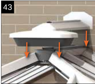
43 Fit the ridge top cap complete with flashing trim and crown cap to the ridge.
